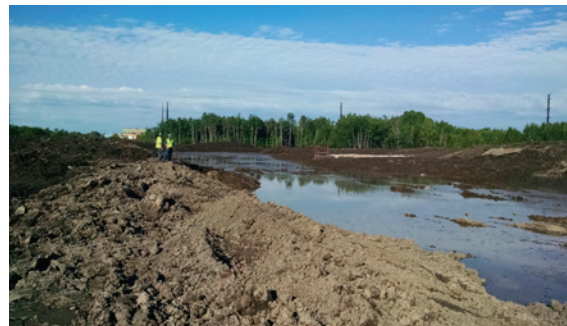
The upland stockpile location of the material gathered from the river. It is being dewatered and is being stored until it can be reused.
